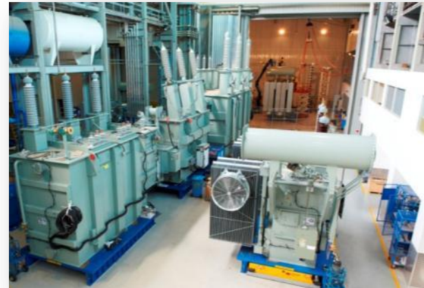
World class transformer plants in Melbourne and Wodonga
